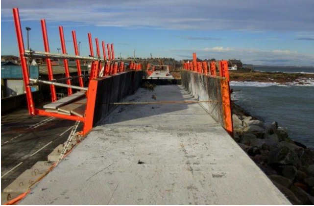
Shutter during construction. The road to the left the sea to the right
