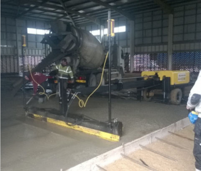
A laser screed could be used continuously without the need for breaks in installation to fix conventional steel mesh reinforcement.
