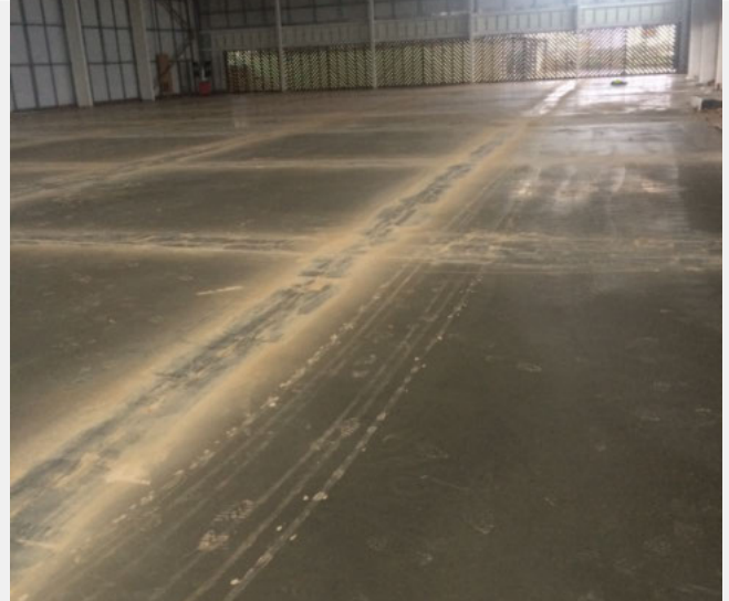
Large areas of pavement could be poured and power floated. Saw cut contraction joints were then made the following day.
