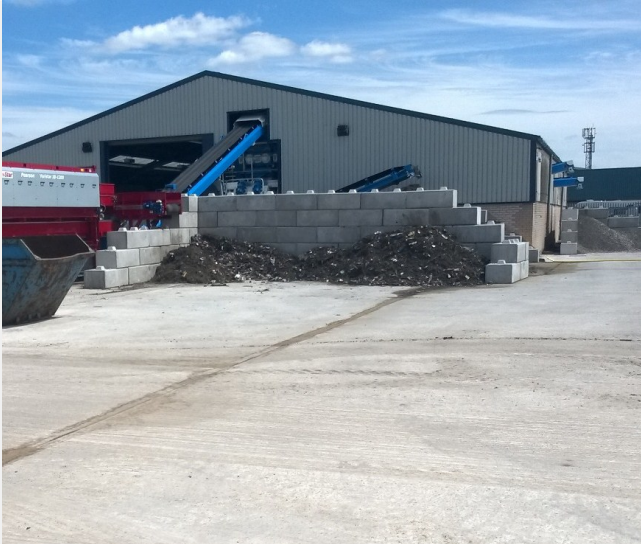
The processing operation exposes the concrete to high levels of road deicing salts that would quickly corrode any steel reinforcement
