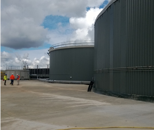
Large areas can be poured straight from the truck without the need for pumping.
